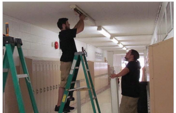
Energy Optimizers, USA updates hallway lighting
